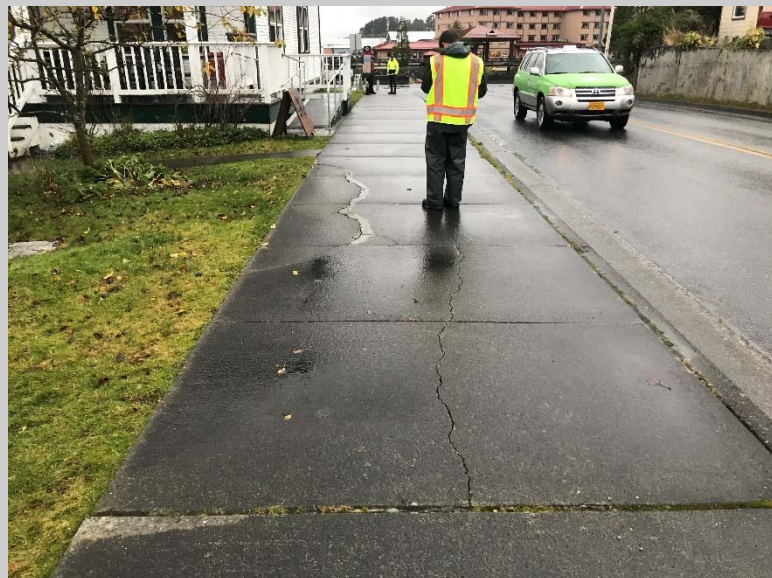
Settlement cracking in the existing sidewalk outside the Beak Restaurant in Section 3.
